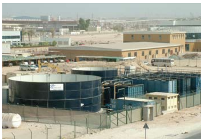
Palm Water's first temporary sewage treatment facilities in Jafza
