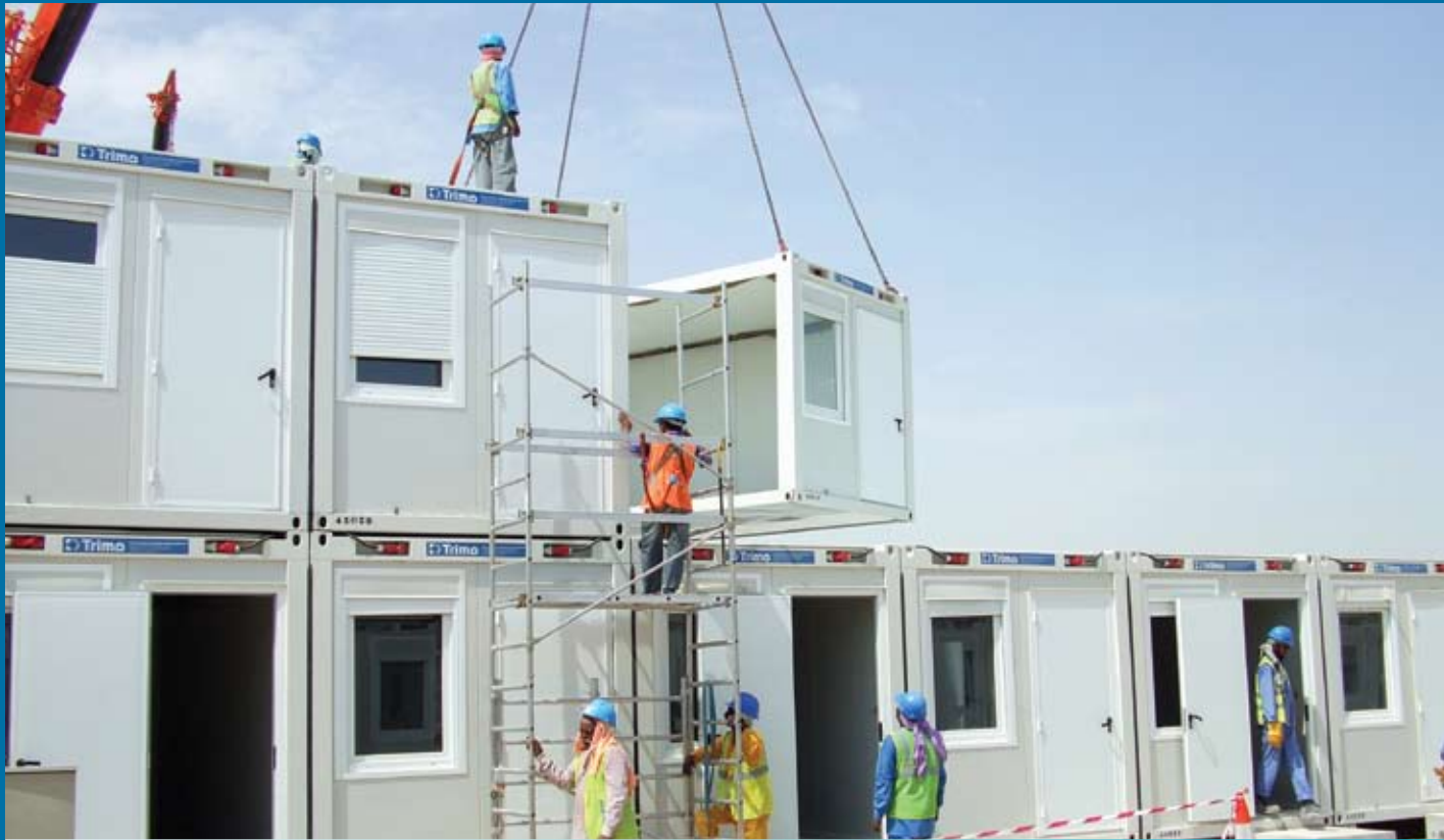
New Labour Accommodation Project at Jafza South (Picture only for illustration purpose)
